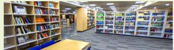
LED Lighting in Library
